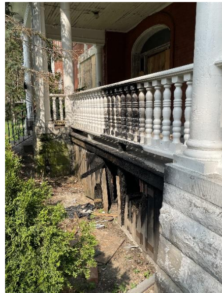
Photo 35: Evidence of fire at porch
