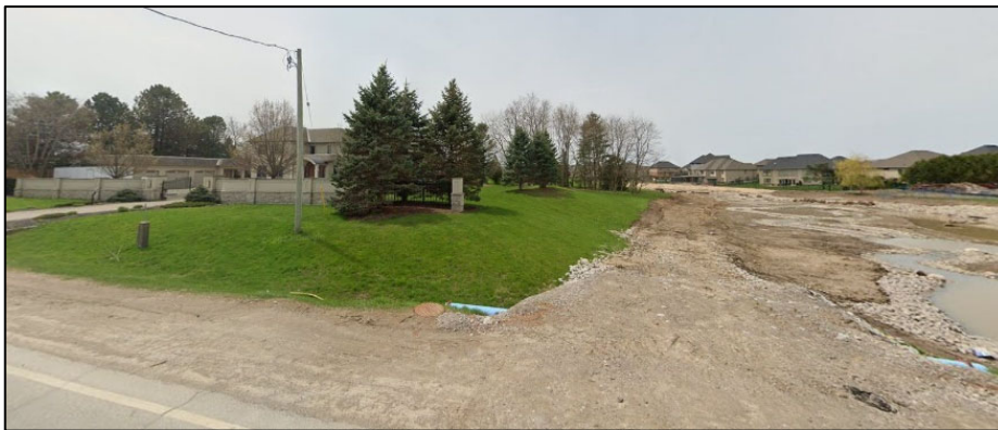
Figure 3. Street view of 3637 Colonel Talbot Road showing creek restoration work (2022) being completed on the Clayton Walk Park tributary (looking west from Colonel Talbot Road).
