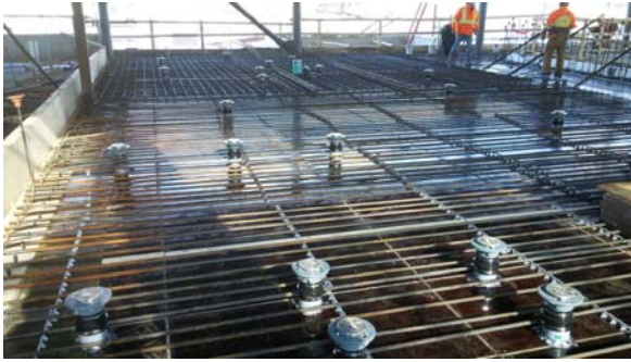
4. Forming for Pool Change Rooms in place with floor drains roughed in.
